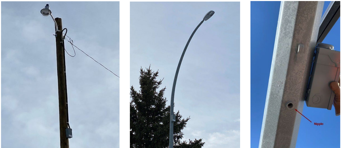
Figure 4 – Wi-fi Device (Left), Security Cameras (Center) and Telecommunication Micro Cell (Right)
