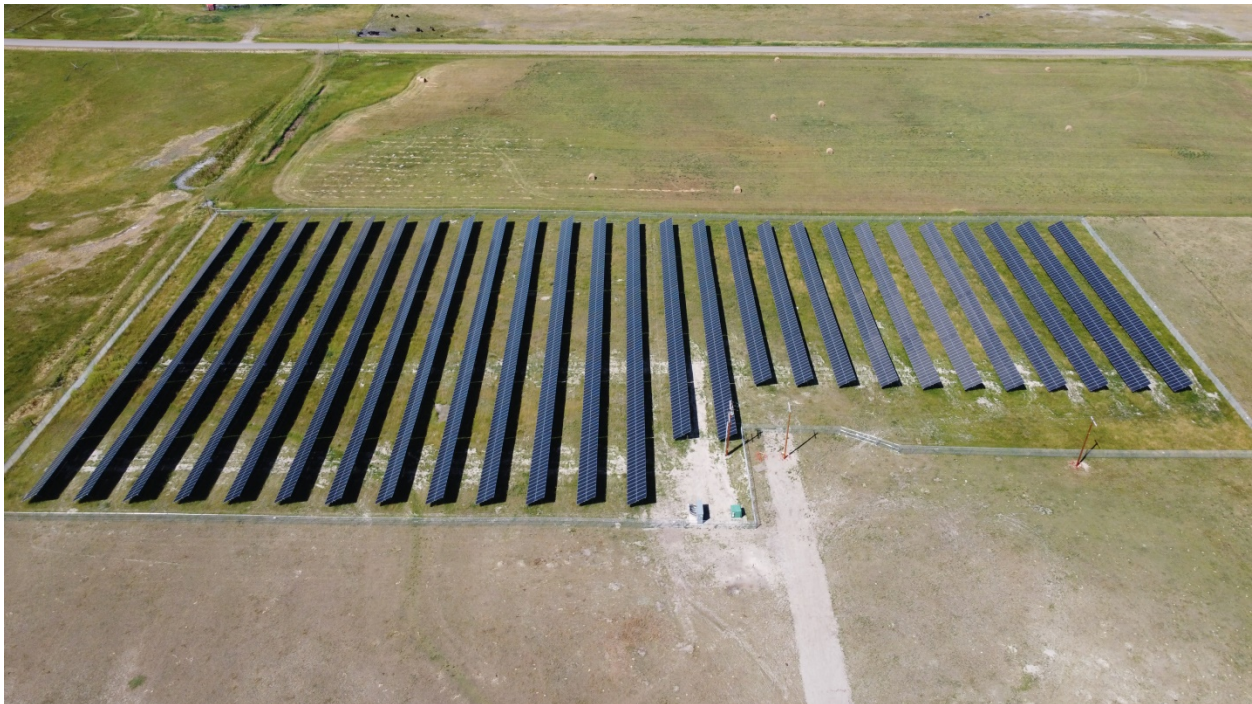
4,752 panels covering 8.5 acres located within the Town of Cardston.
